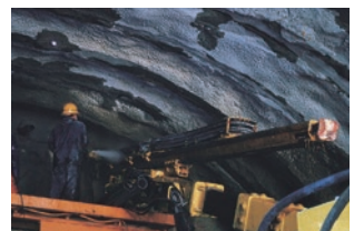
Fore Piling For piling as a reinforced method of tunneling in collapsing overburden.
