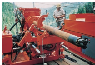
Pipe Roof, Water Service Water Remove, Anchoring It achieves excellent results for drilling of long holes and hard formations using the Down The Hole Hammer. Top-Hammer applications are available.
